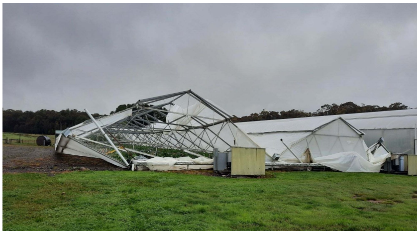
Structural damage at Yendon Gourmet Hydroponics
